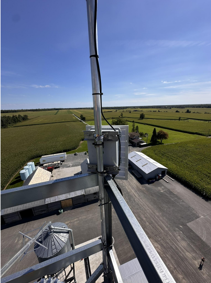
Repeater antenna installation near the top of the grain elevator.
